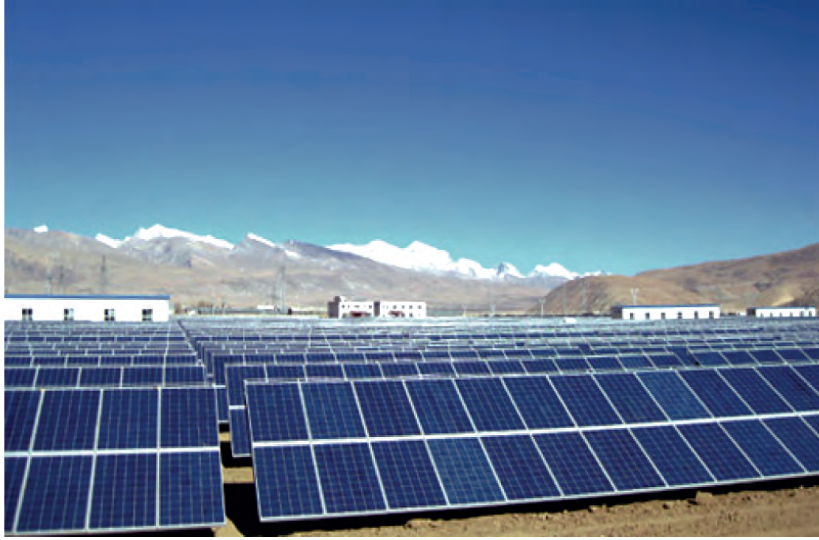
Tibet 10MW Solar Power Plant
